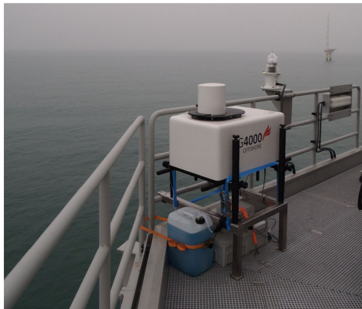
Figure 4: Galion G4000 Offshore scanning wind lidar installed on the transition piece access walkway on Alpha Ventus Offshore Wind Farm Wind Turbine AV07
