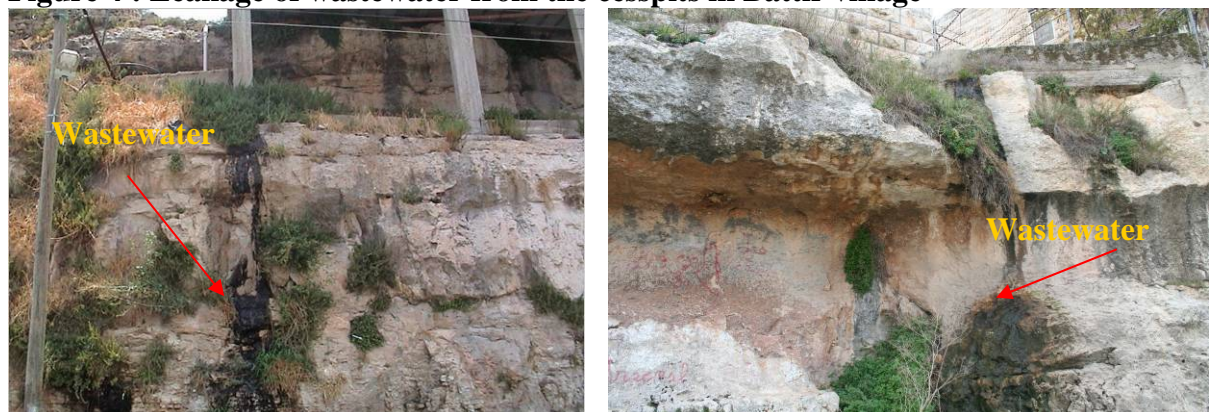
Figure 4 : Leakage of wastewater from the cesspits in Battir village
