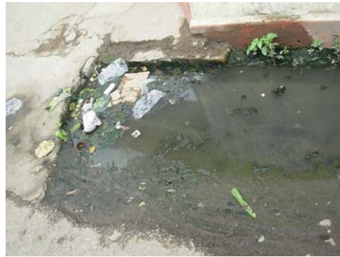
Choked open drains due to waste
