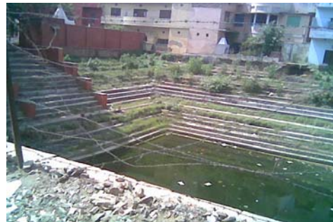
Deteriorated condition of Kunds
