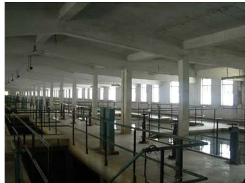
Water Treatment Plant at Bhelupur
