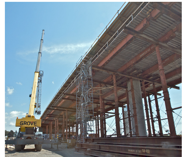
Construction of a bridge on Highway 7 in Whitby as part of the on-going work
