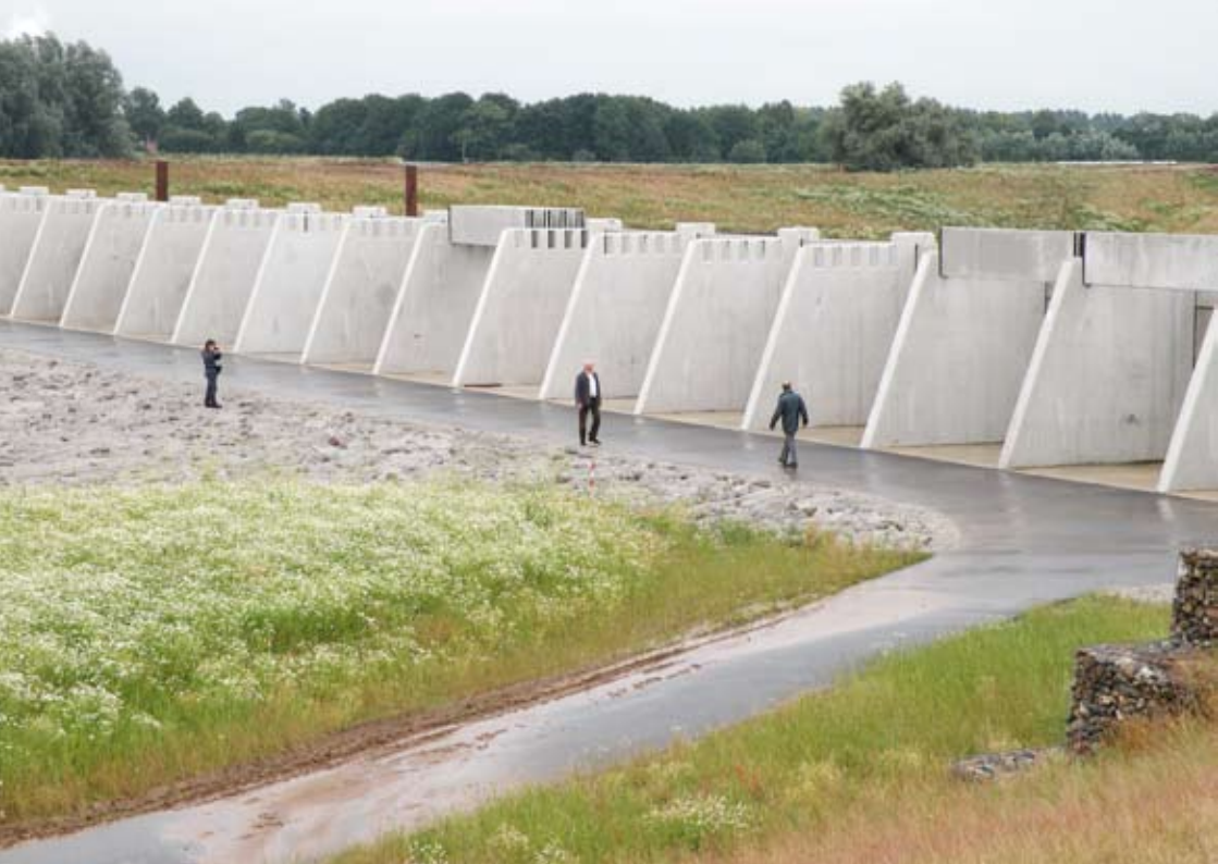
Control device for excess water on the right bank of the rivers Lower Rhine and IJssel.
