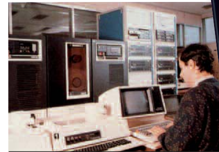
Equipment from the centre national de supervision (National Supervision Center). With SESA, the Group provided the terminals and software for the electronic directory.
