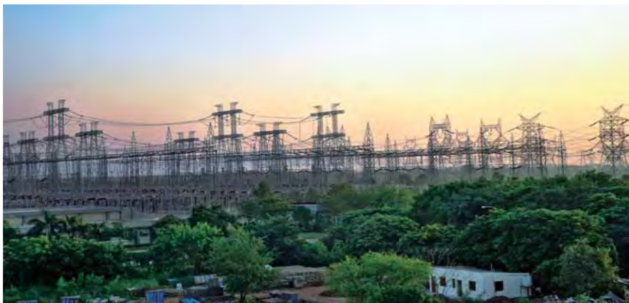
Switchyards are part of L&T's capability in executing projects for power transmission and distribution
