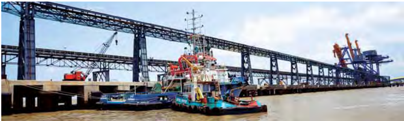
Ports are part of the wide portfolio of major infrastructure projects built by L&T.
