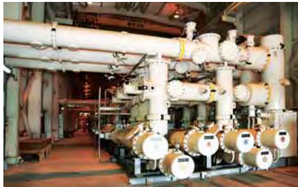
400 kV GIS Switchyard, NTECL Vallur of 3 x 500 MW Thermal Power Plant
