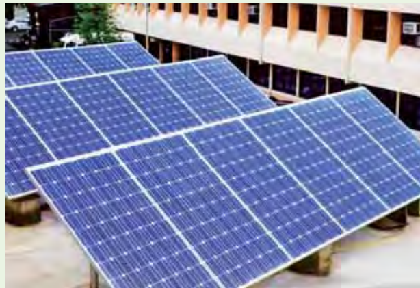
Solar PV panels installed at Powai campus
