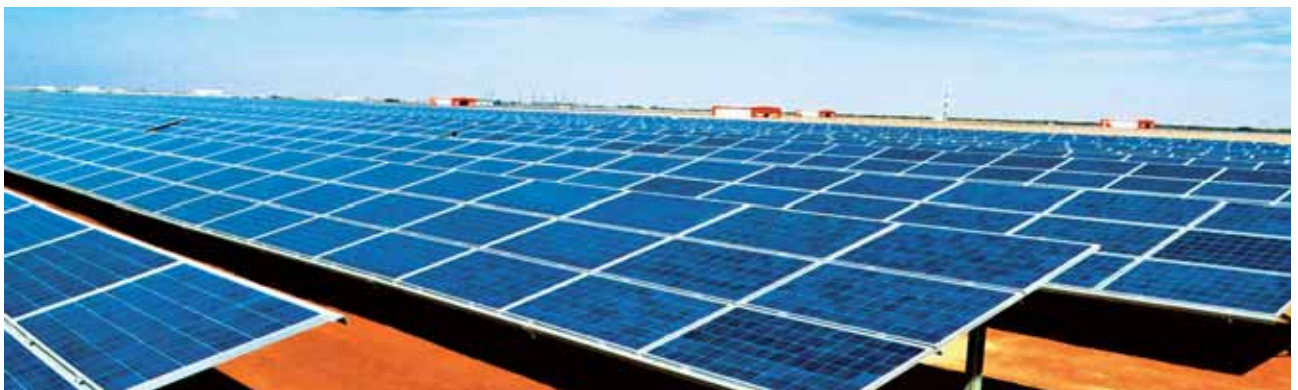
India's largest solar plant built by L&T in Rajasthan.
