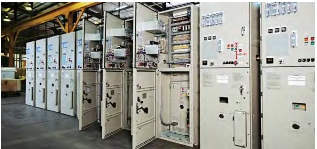
Medium Voltage Switchboard Panels of Tamco, an L&T subsidiary.
