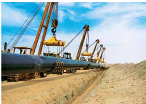
Habshan-Ruwais-Shuweihat Pipeline being executed on an EPC basis in Abu Dhabi. L&T has constructed over 4,000 km of pipeline across some of the world's toughest terrain.
