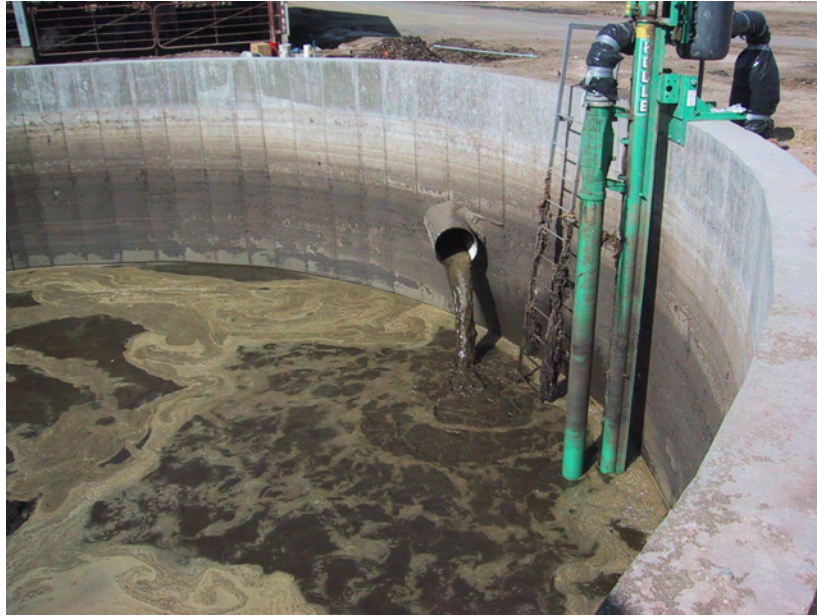
Typical Manure Sump with Chopper Pump
