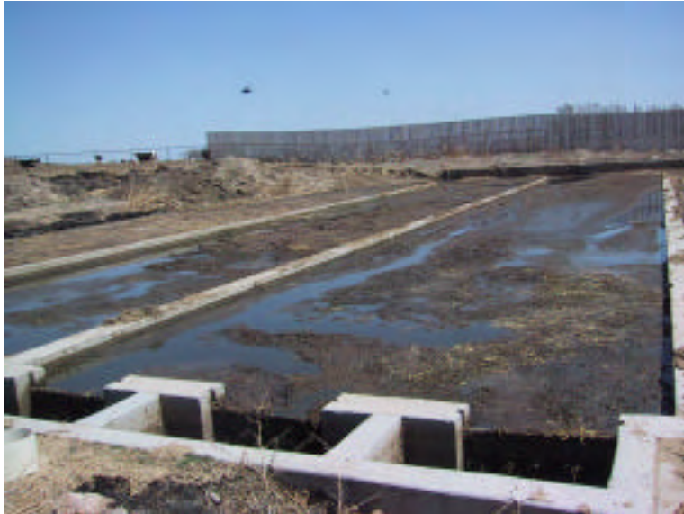
Floating Solids on Top of Gravity Separator
