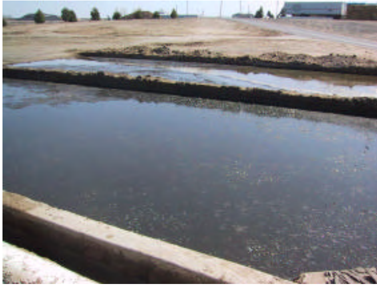
Gravity Separator with Anaerobic Decomposition of Organic Solid
