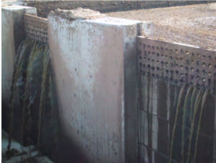
Weeping Wall with Clogged Holes
