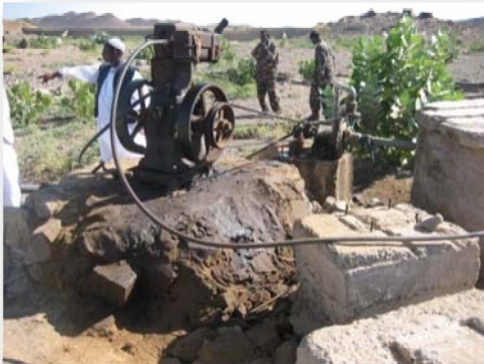
Fig.9: Three years old diesel pump leaking oil
