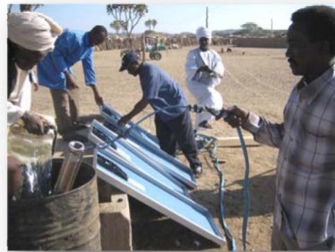
Fig.10: Testing the solar-powered submersible pump
