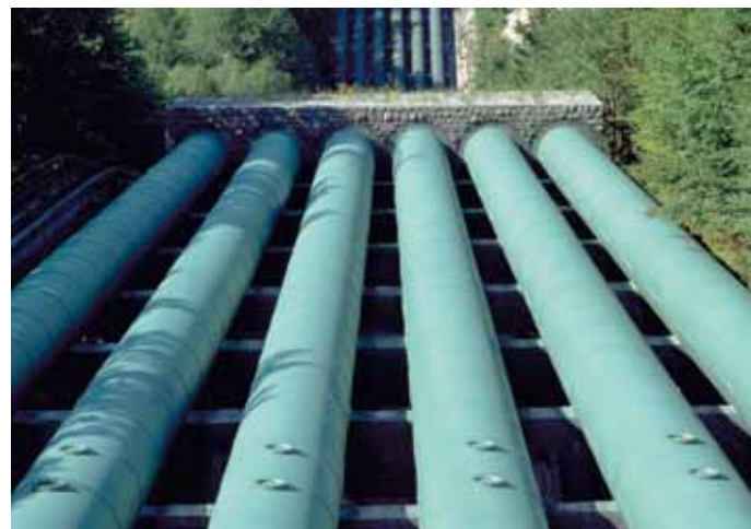
The surge chamber with its six huge power pipes high up on the mountain is the visible hallmark of the Walchensee Power Station. Together they have a weight of around 3,600 tons.
