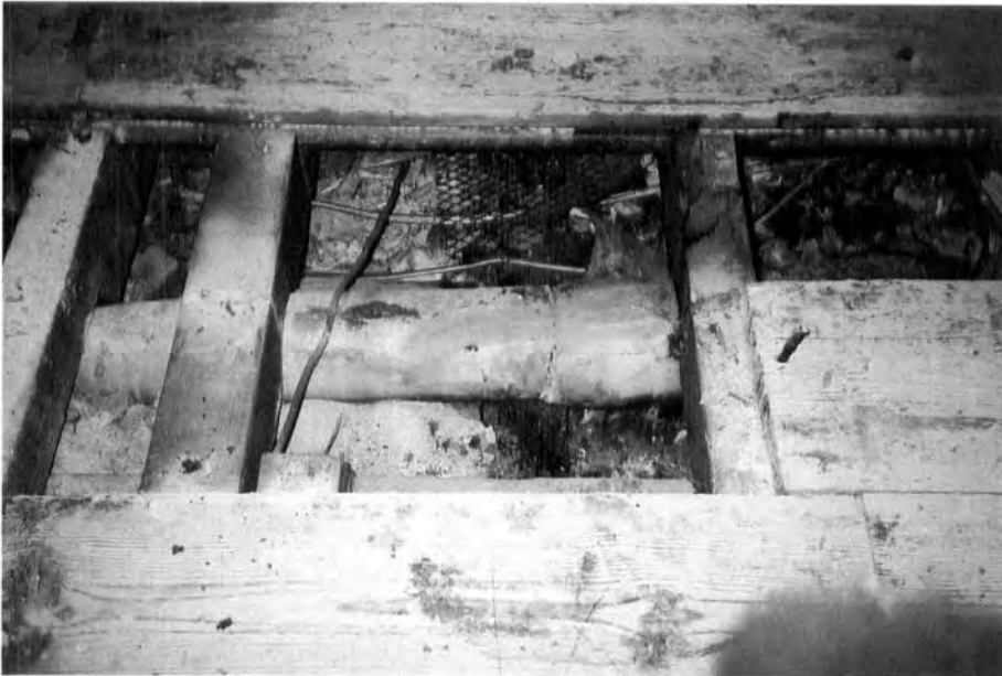
The bent and broken lead pipe which has now been replaced.
