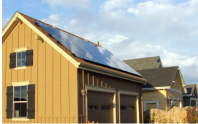
Residential photovoltaic installation in Lafayette, Colorado
