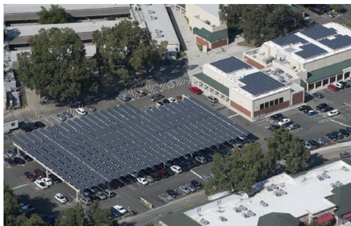
Commercial photovoltaic installation on commercial building and parking shade structure in San Ramon, California
