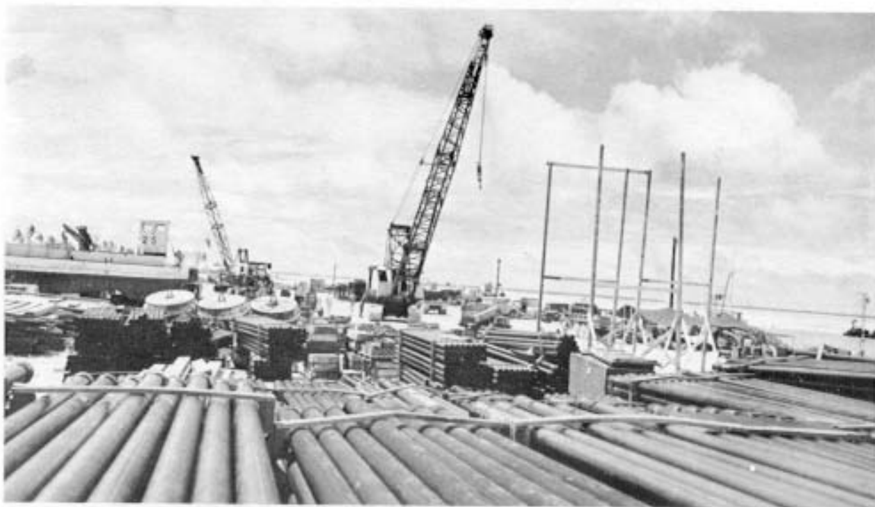
Figure 6. Christmas Island harbor area showing pipe for Army Engineer pipeline construction, DOMINIC.
