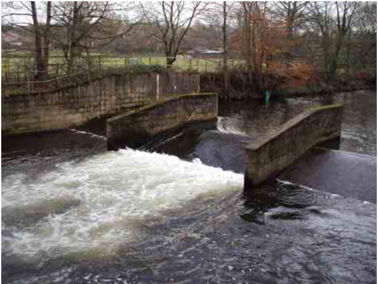
Figure 2 | Gauging station at Marple Bridge
