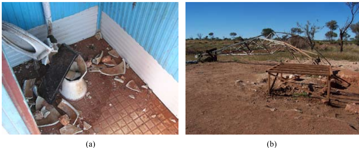
Figure 7.3: (a) Toilet on an Aboriginal settlement near Warburton in the Ngaanyatjarra lands (WA) that has been damaged by camels (image courtesy P. Morrison); (b) Windmill at Blackstone in the Ngaanyatjarra lands (WA) that has been damaged by camels.
