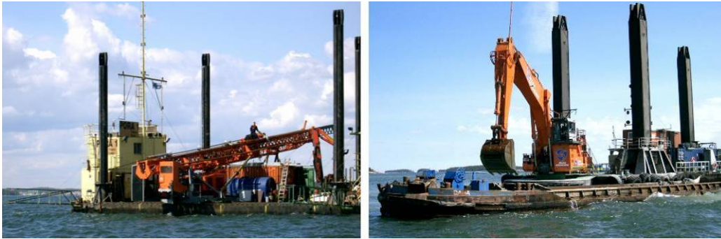
Figure 0-6 Example of drilling and blasting barge (left) and a dredging barge (right) working on the Vuosaari harbour project, year 2004.
