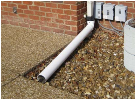
◀ By at least disconnecting downspouts from being channelled directly to the stormwater system, stormwater runoff can often be handled on site.
