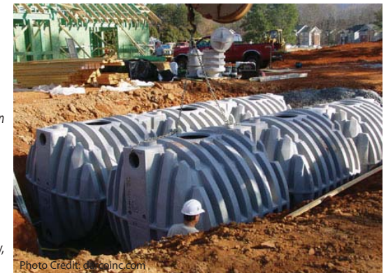
► This underground cistern will hold 12,000 gallons. Typically a 1,100 gallon cistern may capture 80% of the runoff from a 1,000 sq.ft. roof. (Source: Green Infrastructure Master Plan, Nashville Davidson County, Metro Water Services)
