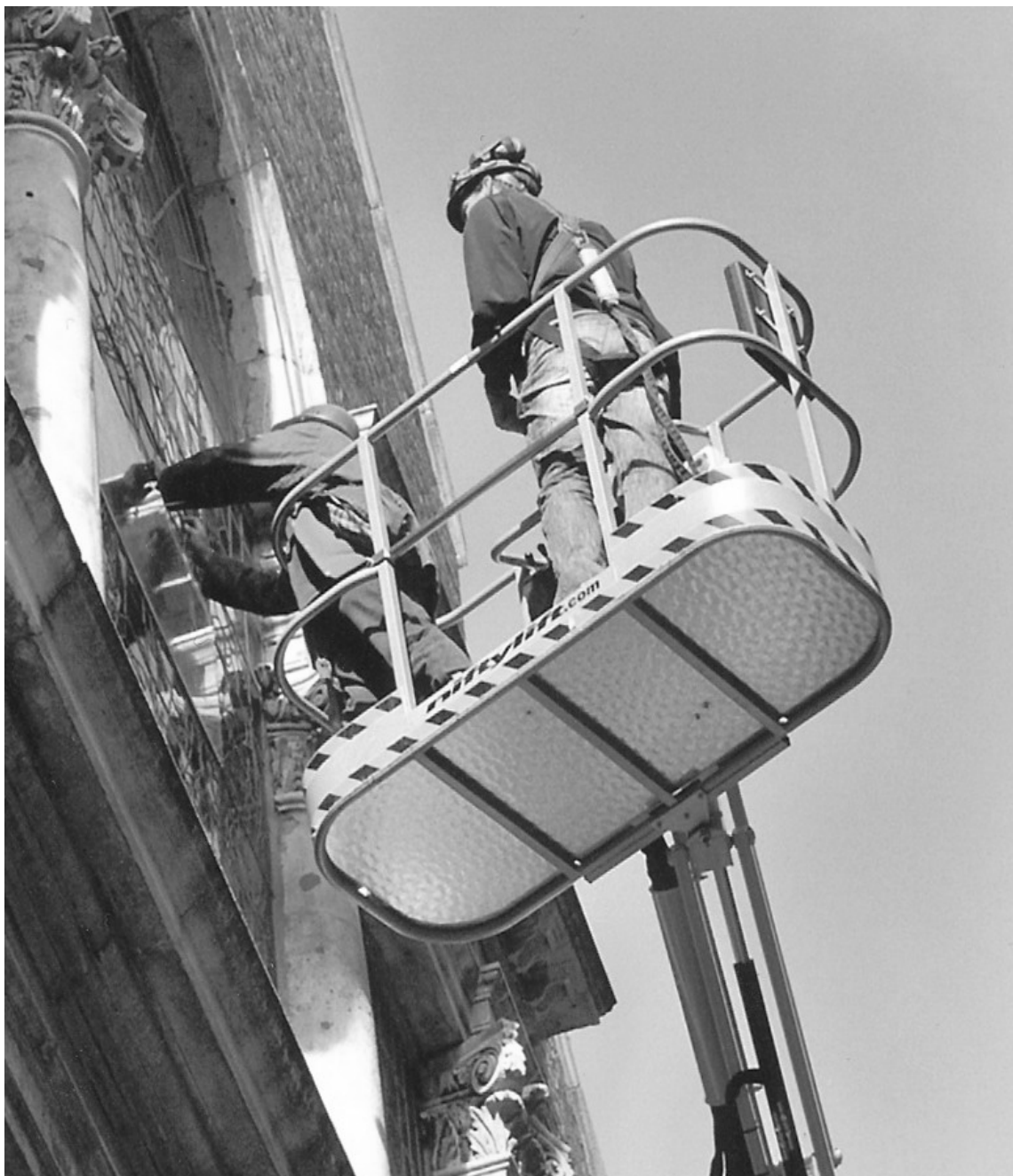
Repairs to the East window: the cherry picker crane carries the stained glass expert up to the window
