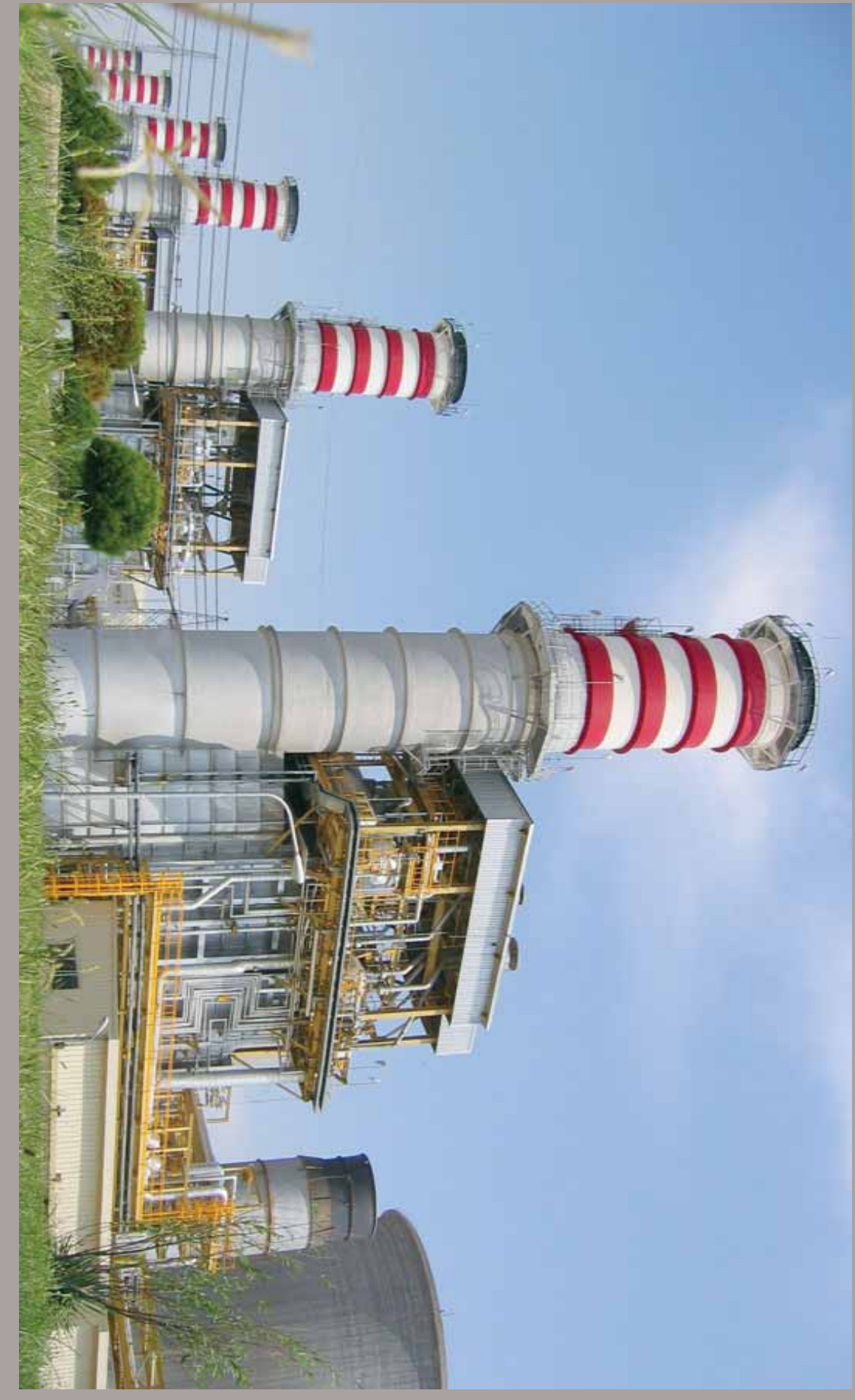
FARS CCGP Power Plant
