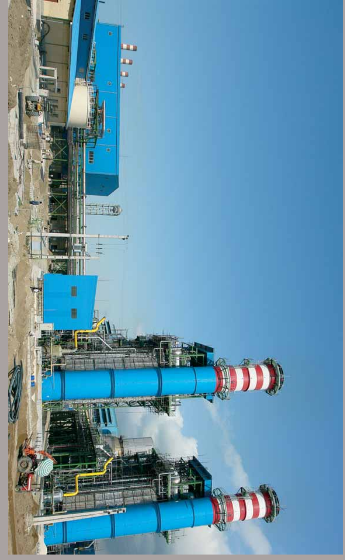
NEKA CCPP Power Plant
