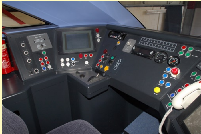
ABOVE: 'Javlin' cab layout, incorporating left hand power/brake controller, plus full TVM430 cab-signalling and traditional radio and AWS/TPWS equipment.
