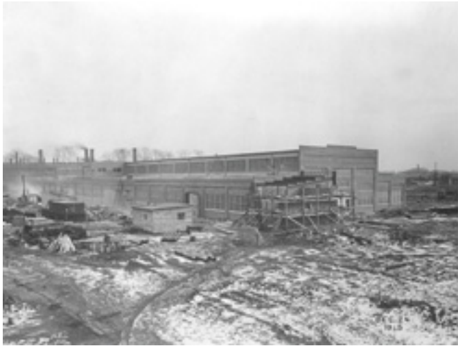
Construction of this building at the West Avenue facility, for the manufacture of shells, started in November and completed on December 24, 1915.
