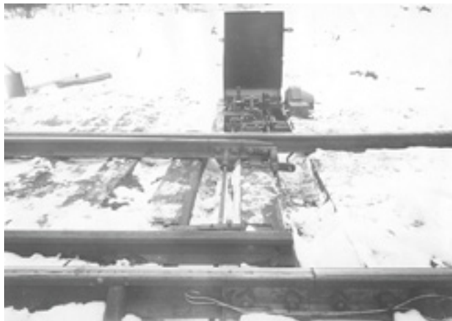
Model 2 Electric Switch Machine at Eau Claire, Wisconsin.
