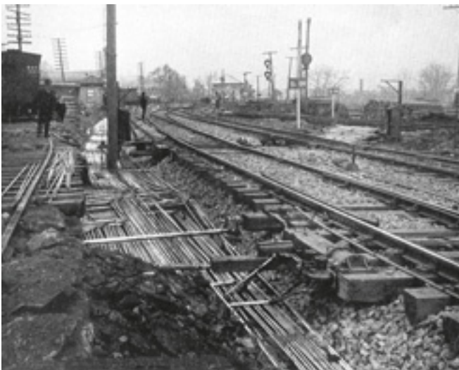
The pneumatic interlocking installed in 1900 at Wayne Jct., PA required thousands of feet of underground pipe.
