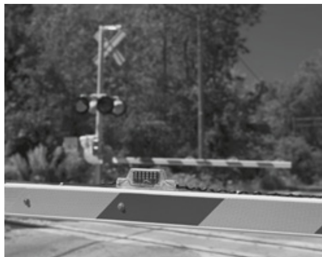
AURORA LED Crossing Signal and Gate Arm Lights (1997).
