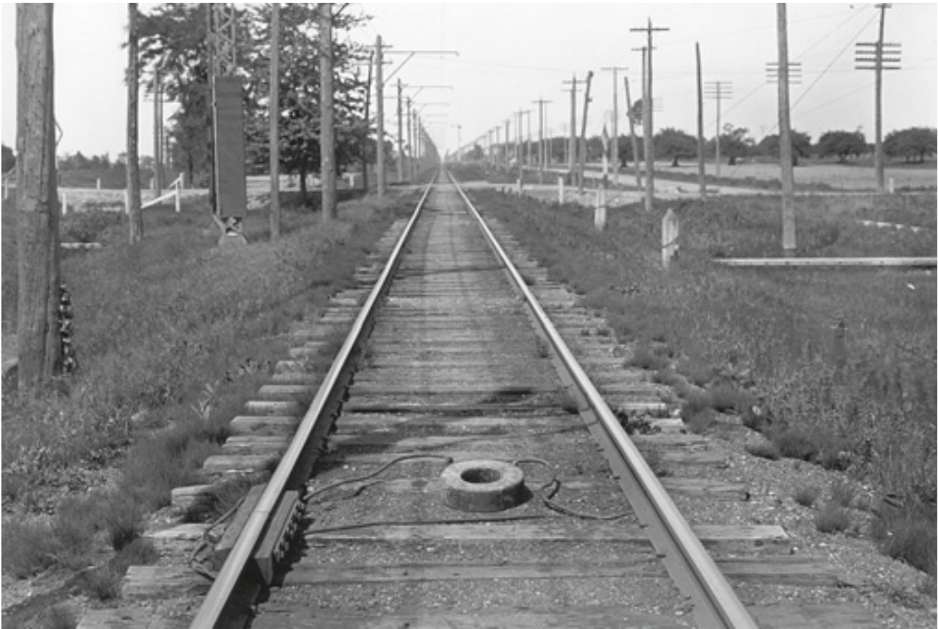
An "ironless bond", part of the Young system of a-c block signaling.
