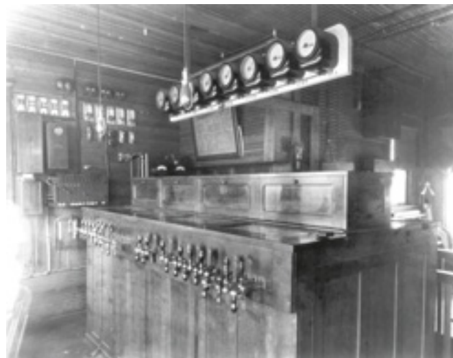
In 1904, this GRS electric interlocker was installed at East Norwood, Ohio, on the B&O Southwestern R.R. to replace the original 1889 Taylor machine.
