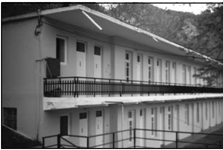
Figure 6. An old complex of rooms to let, without heating facilities open only in summer
