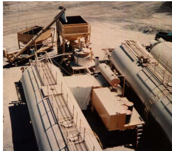
Figure 3-2: Asphalt Rubber Production Set Up At AC Plant
