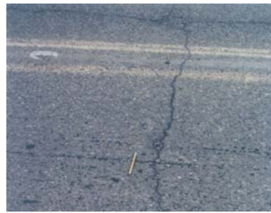
Photo 2. Low Temperature Cracking
