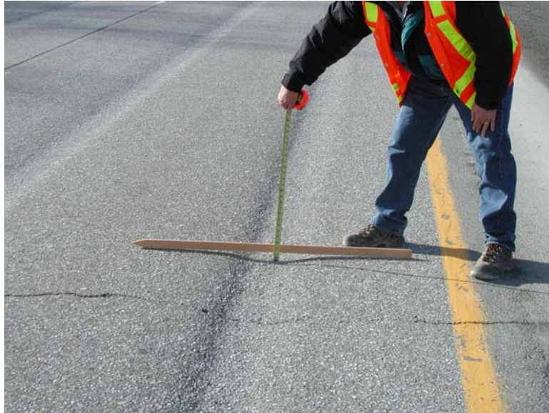
Figure 16. Raveling Distress due to Studded Tire Wear
