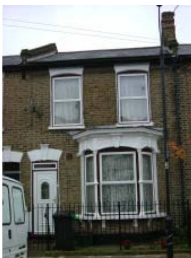
Replacement windows in upvc are different in appearance to the characteristic timber framed sliding sash windows seen across the conservation area. The door is also of non-traditional design and materials and is set further forward than other doors.
