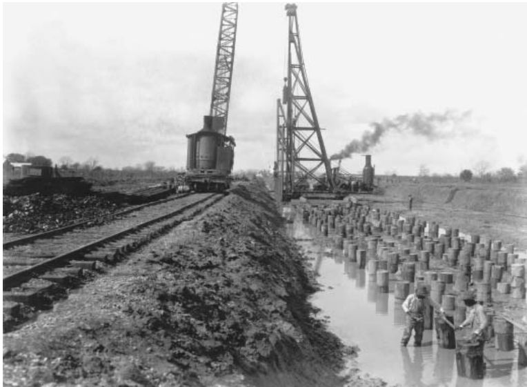
Thousands of wooden pilings were driven to provide a reliable foundation for the spillway structure.
