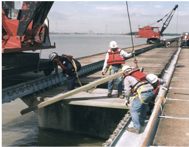
In opening the spillway, each timber is individually lifted and placed atop the structure.
