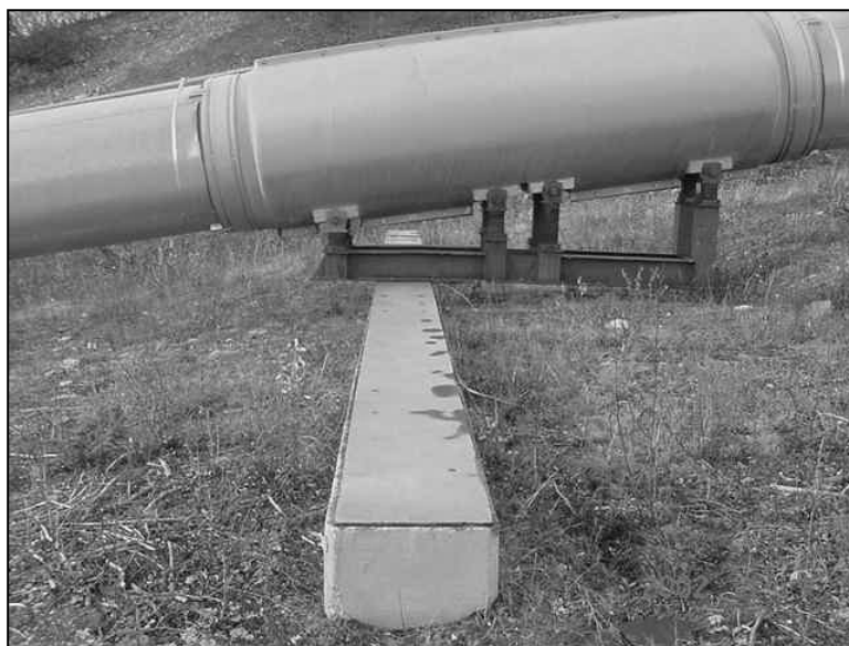
Figure 3. Typical special configuration bent on a concrete grade beam: Note offset shoe position by design to accommodate pipe movement in this case to the left.
