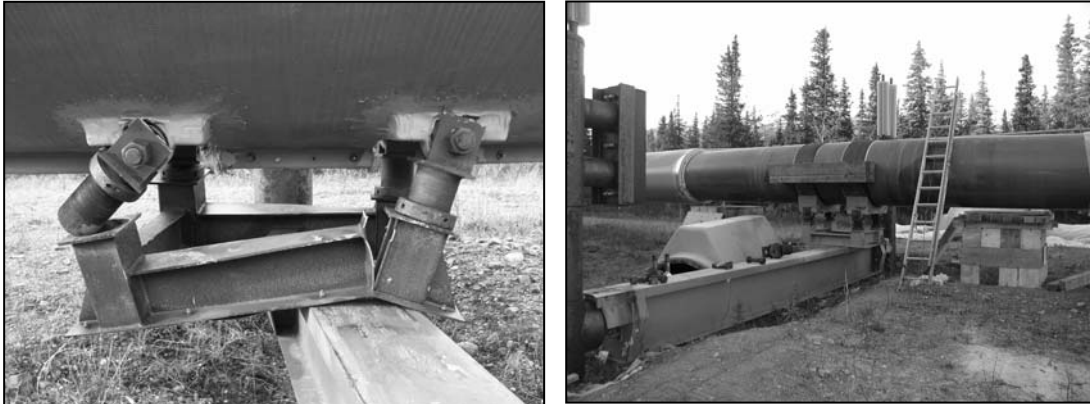
Figure 5. Post-event shoe damage (left) and pre-startup repair (right) on the seismic bent immediately south of the Denali Fault. Note the temporary shoring beneath the pipe used during repairs (right side of picture), the bumper beam on the pipe clamp (center), and the impact absorber on the VSM (far left side of picture).
