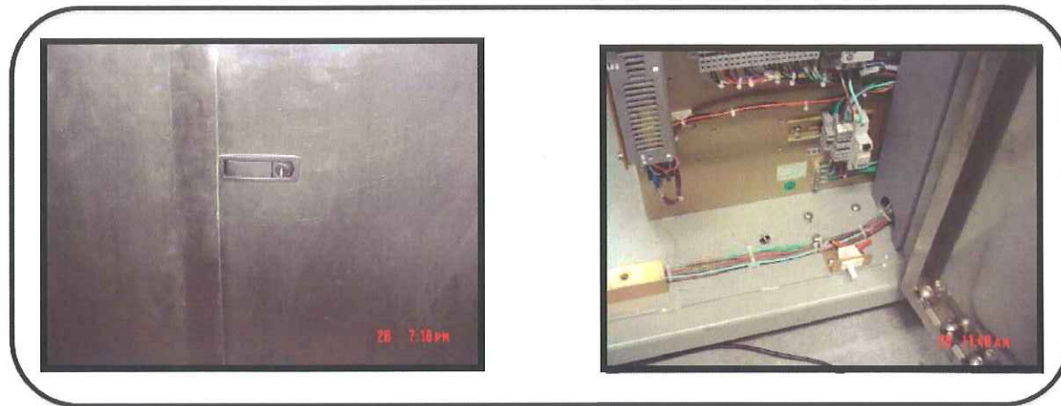
Figure 8-22: Access Panel Door and Door Interlock
