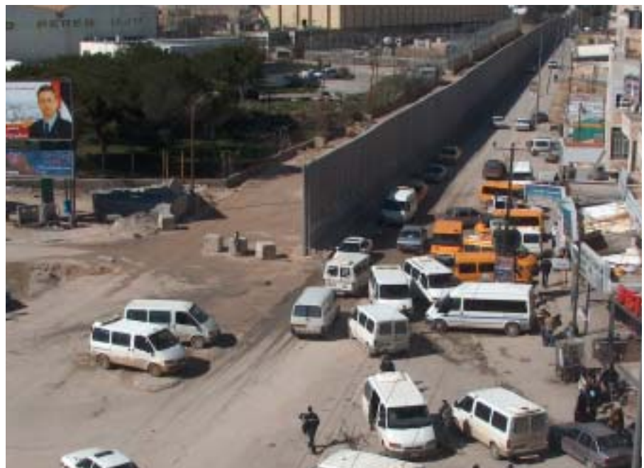
The Barrier under construction down the middle of the road in Ar Ram.
