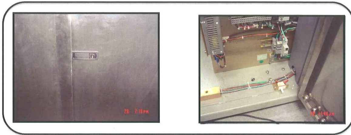
Figure 8-22: Access Panel Door and Door Interlock
