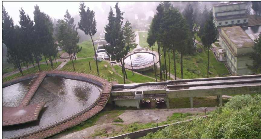
Selep WTP with pre-sedimentation tank in left foreground
