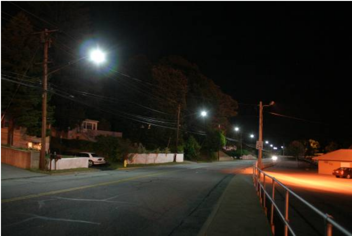
Figure 3. Induction street lighting demonstration (Meridian Street)
