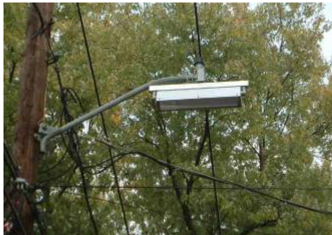
Figure 6. Fluorescent luminaire with flat lens
