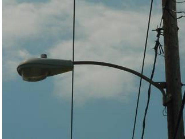
Figure 3. Existing HPS luminaire
