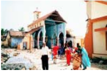
Kerala Manakudy Church damaged
