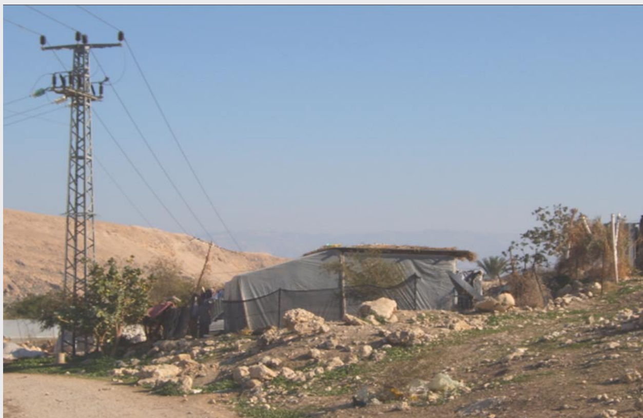
Power lines passing over Al Jiftlik village to provide electricity to nearby Israeli settlements. Photo by OCHA, 2007.
