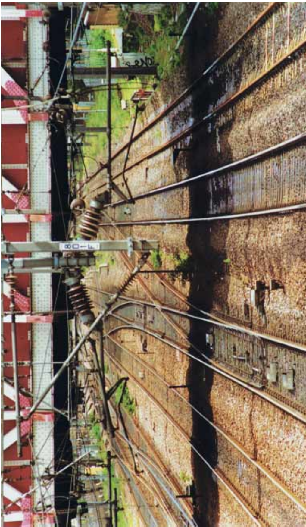
Plate 14: View towards Paddington. Taken from Gantry 8 with the camera placed directly above the red aspect of SN109. The lines are numbered 1 to 6 from right to left. SN109 applies to Line 3.
