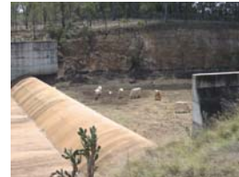
Gordonbrook Dam showing lack of water at the crest of the spillway
