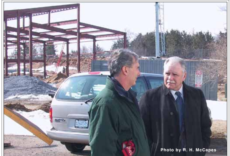
Charles Wenderoth, PIADC Facilities Engineer, briefs USAHA president Robert Frost on construction of new power plant during a review of PIADC facilities, March 2003.
