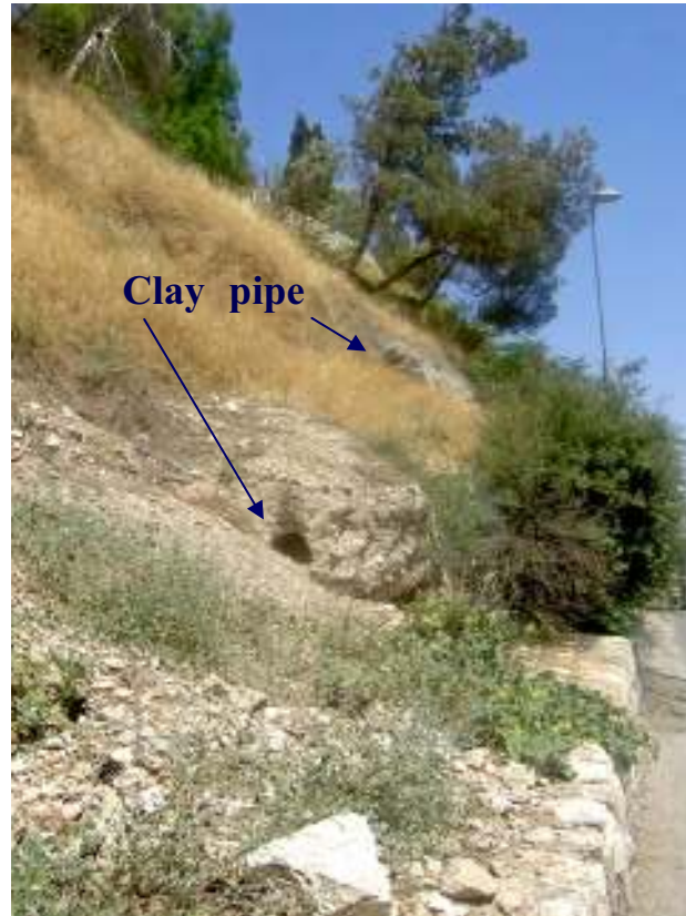
Figure 69. The lower aqueduct located on the southern side of Mt. Zion, partly broken and showing the installed Ottoman clay pipe.
