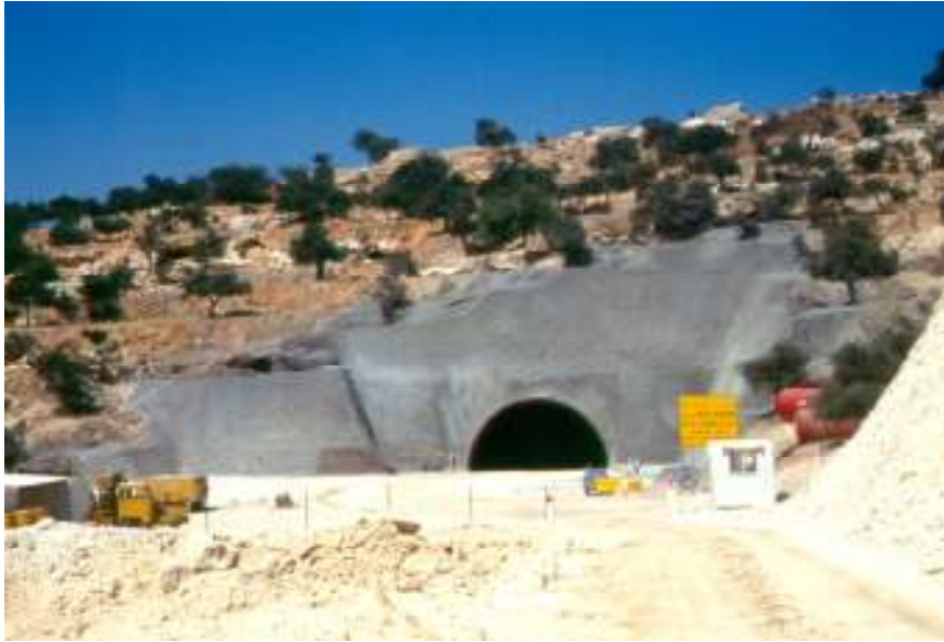
Figure 41. View of the north portal of the Gilo Short Tunnel in the Kefar Sha'ul Formation during construction.
