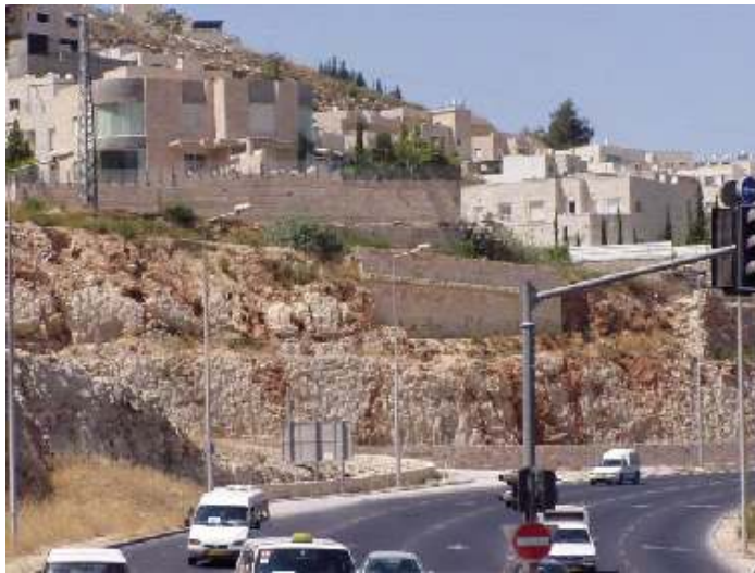
Figure 28. Karstic holes in the Amminadav Formation seen as brown patches of red-brown soil filling. Herzog Street.
