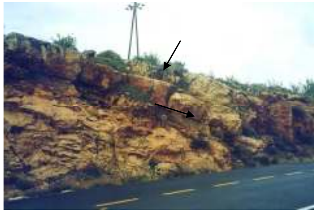
Figure 20. Dip slope failures in road cut.
