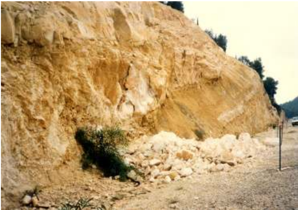
Figure 19. Rock fall in roadcut in the Moza Formation, Jerusalem – Tel Aviv highway.
