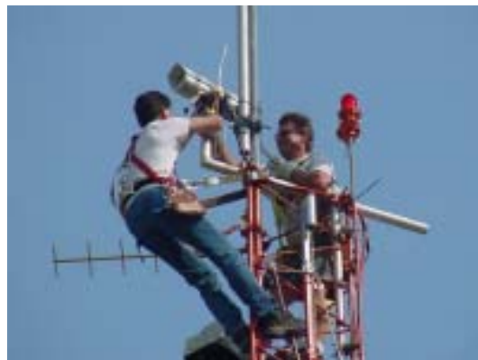
Figure 4. Camera installation on communications tower.
