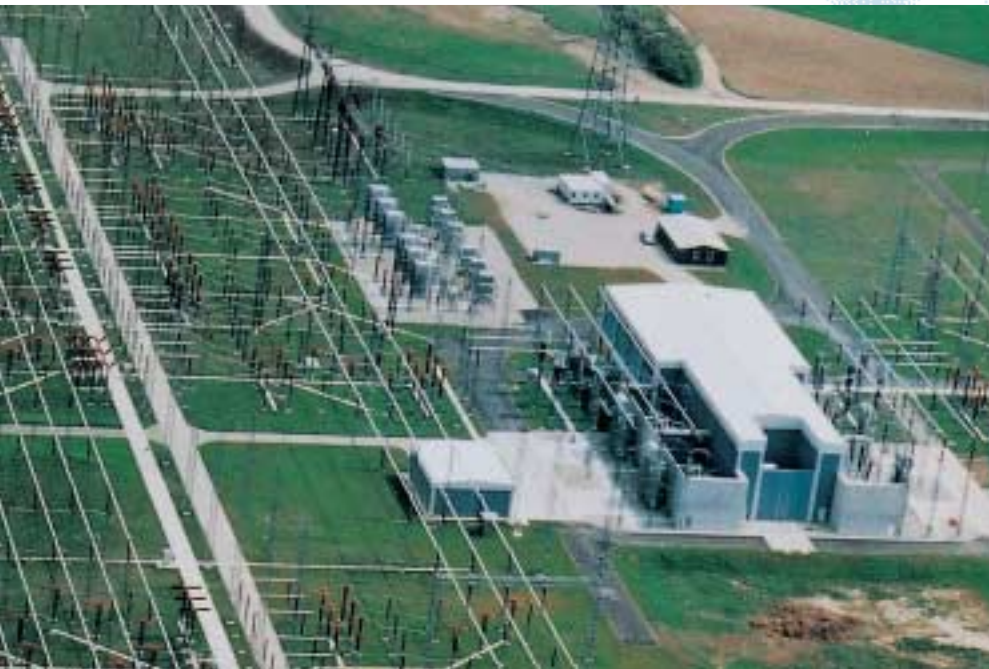
Fig. 2-3: Back-to-back converter Station Vienna Southeast
