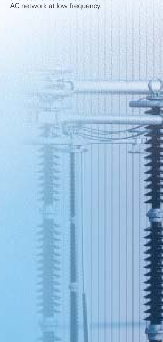
Fig. 5.4.2-1 DC filter of Guangzhou/China
