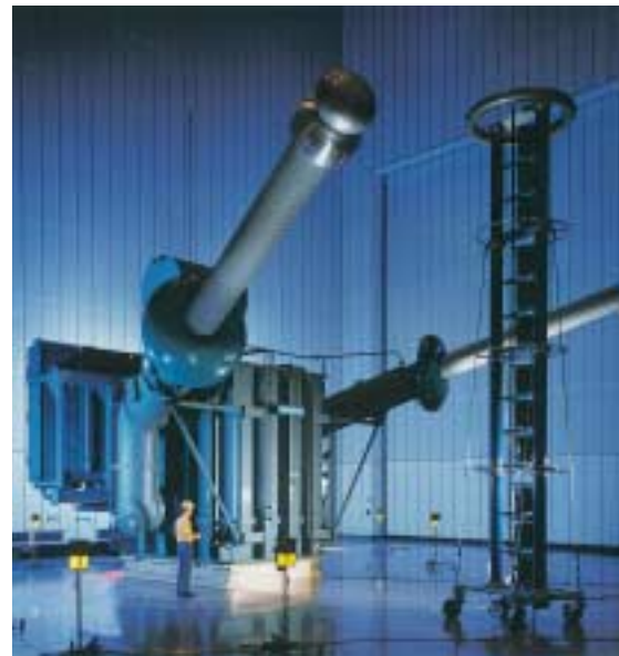
Fig. 5.3-1: Oil-insulated smoothing reactor – Three Gorges project
