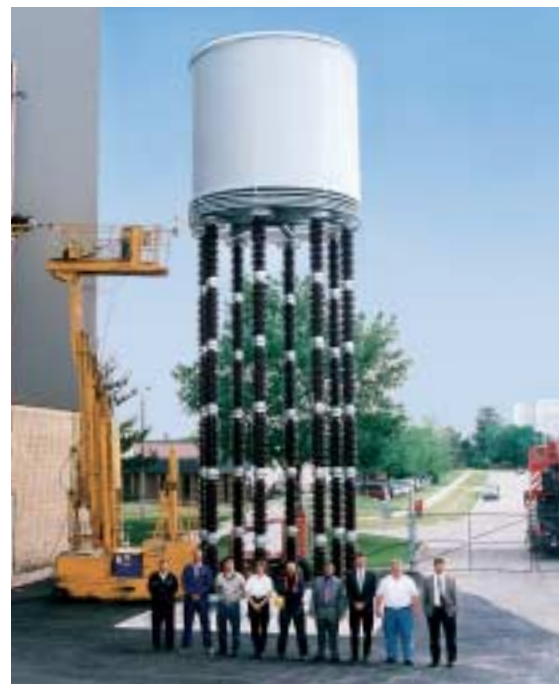
Fig. 5.3-2: Air-insulated smoothing reactor – Tian Guang project
