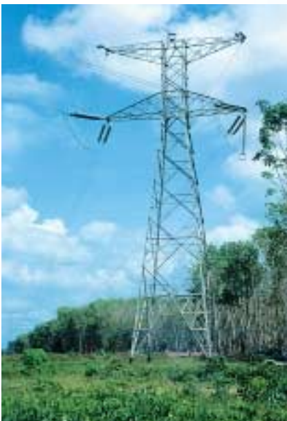
Fig. 5.6.1-1: DC transmission line (bipolar tower 300-kV link)
