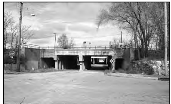
Concrete railroad bridge over South 7 th Street, located north of Pacific Street, DO09:0066-008
