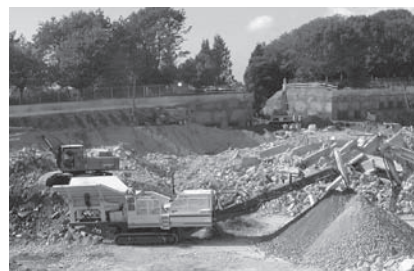
Demolition of the old reservoir and on-site separation of concrete and rebar – Sept 2002
