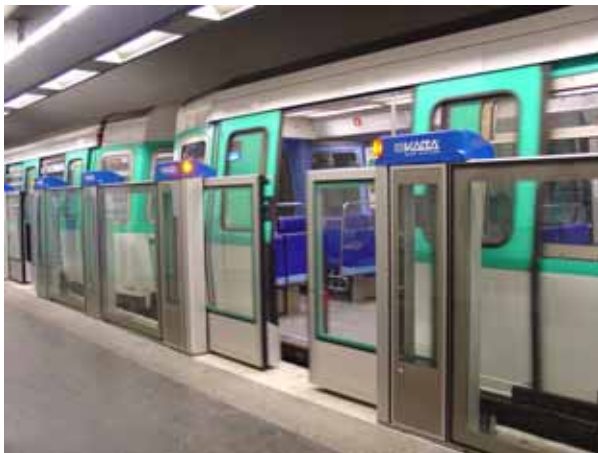
PSD half-height – platform 1 Station Invalides installed and in test operation since March 2006
