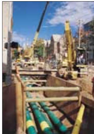
1 Construction on York Street, extending utility service from the Central Power Plant to the new School of Art
