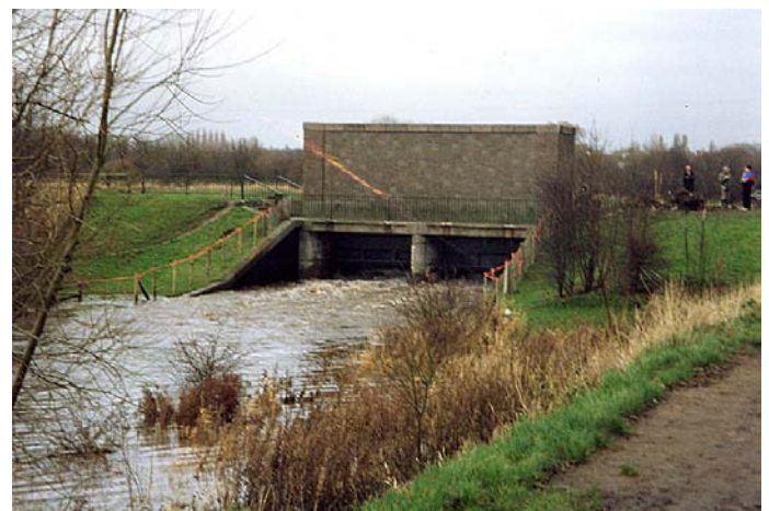
Figure 5: Floodwaters being released from the Mersey into Sale Water Park through the basin inlet near the Jackson's Boat Public House.
