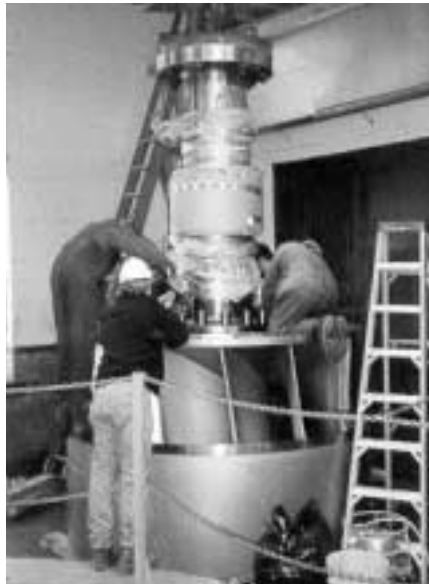
Through upgrades, Great Lakes Power increased its installed hydroelectric capacity by more than 3 percent. In this photograph, workmen are installing a new runner at the 54-MW MacKay Generating Station Unit 2.
