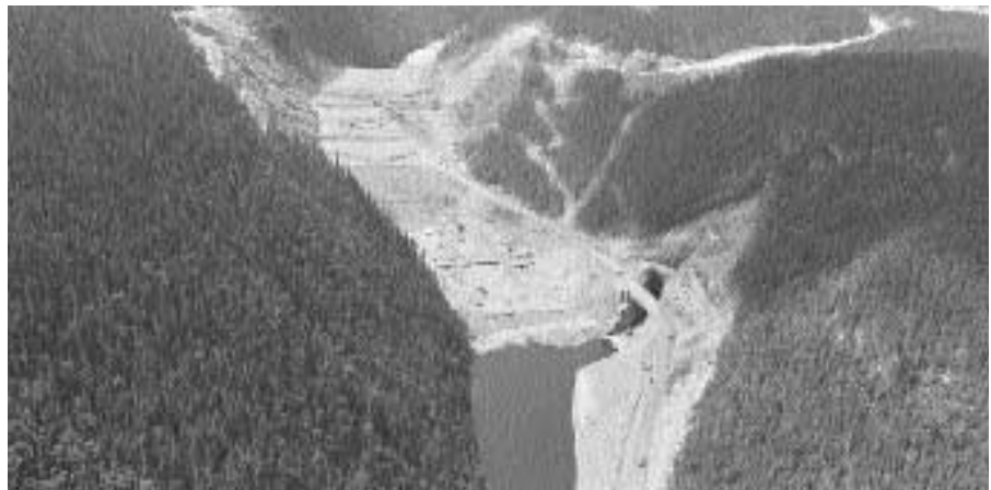
The 882-MW Sainte-Marguerite-3 hydro plant (shown in this photograph), now under construction, is the most important of numerous projects Hydro-Québec has under way to maintain, optimize, and restore facilities and add new ones.
