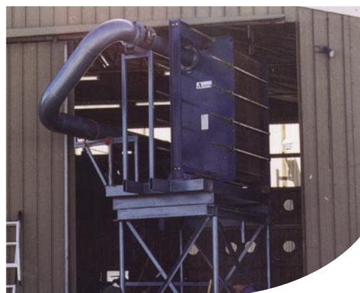
New plate heat exchanger condenser and stand
