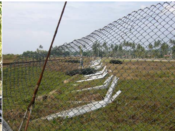
Photo 2 Damaged chain link fence which is 200m inland
