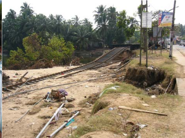
Photo 10 Scouring damage to the foundations of the railway at Ambalangoda
