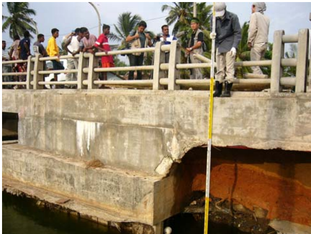
Photo 7 Damaged concrete handrail of the bridge
