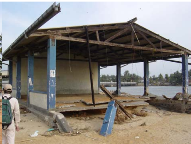
Photo 14 Concrete floor damaged by the tsunami lifting force
