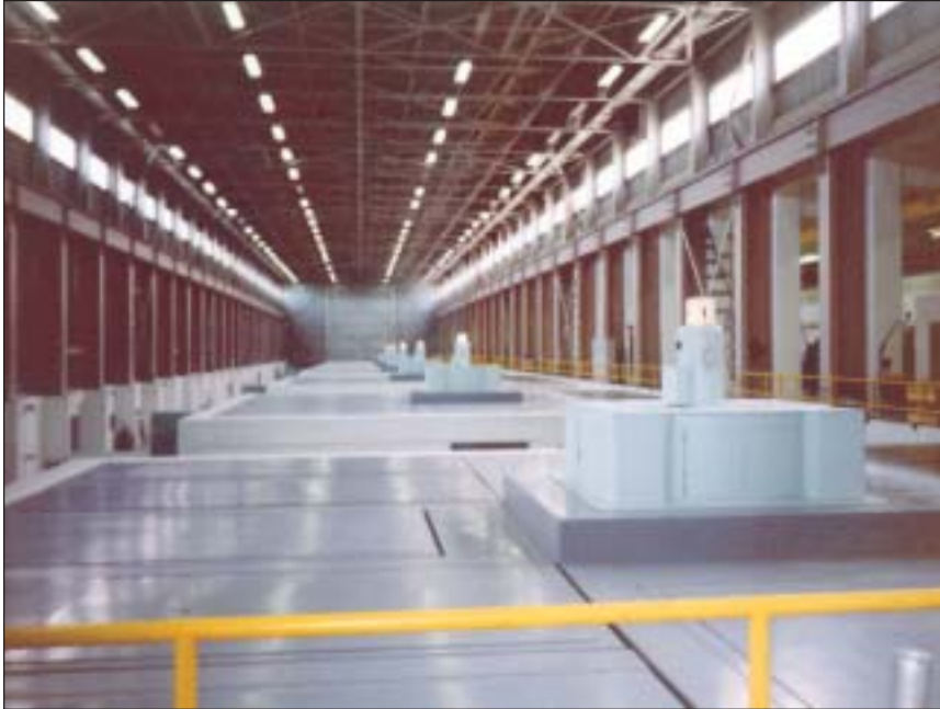
The interior of the Kelsey Generating Station's powerhouse
