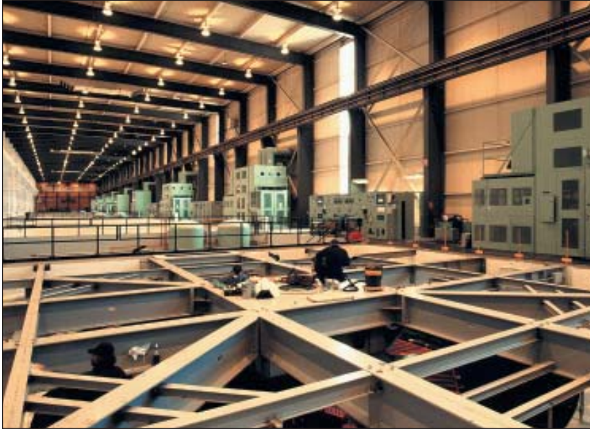
Inside Kettle Generating Station's powerhouse, maintenance work on the turbine generators ensures they will operate to maximum efficiency.
