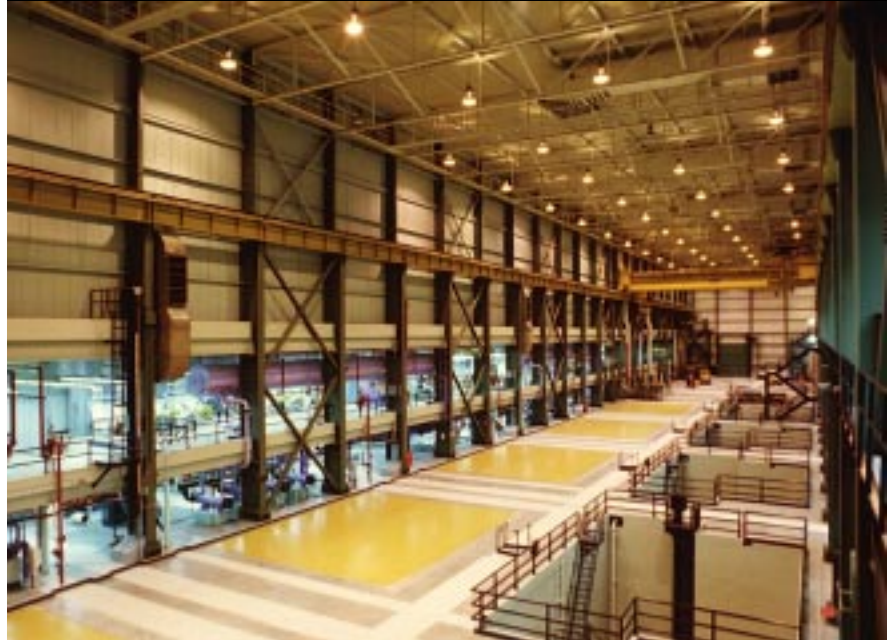
The interior of the Jenpeg's powerhouse.
